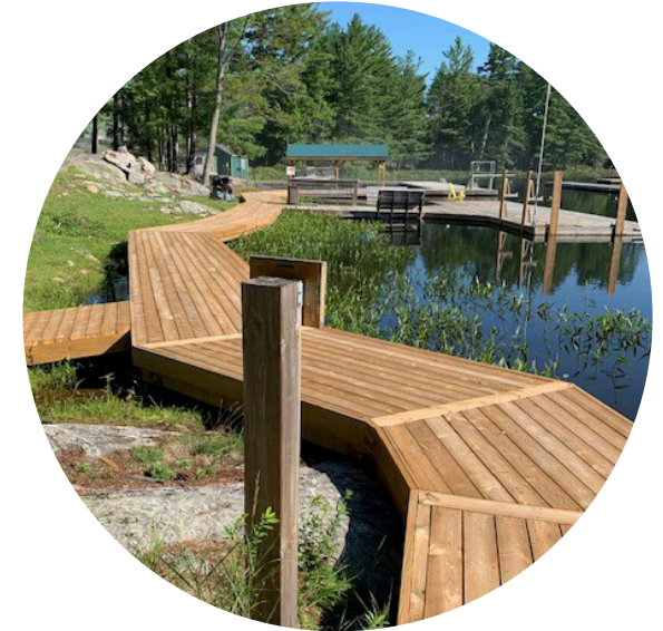
New lengthwise decking along the waterfront gives wheelchair users an easy ride to and from various waterfront activities.
